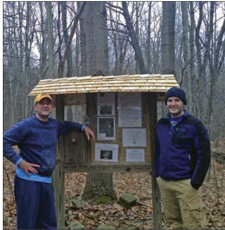
Local residents Ben Farr and his dad volunteered their time on Christmas Day 2015 to replace the roof of the kiosk Ben built for his Eagle Scout project, years ago, at the Ellis Hollow Nature Preserve.
